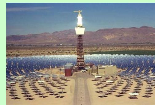
Solar Power Tower
