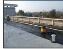
Parapet wall height extension fall protection system
