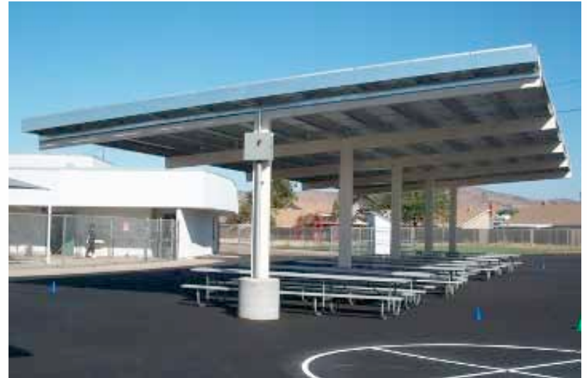
The County's first CREB-financed solar PV project: a 283 kW shade structure at Hill Creek Elementary School in Santee
